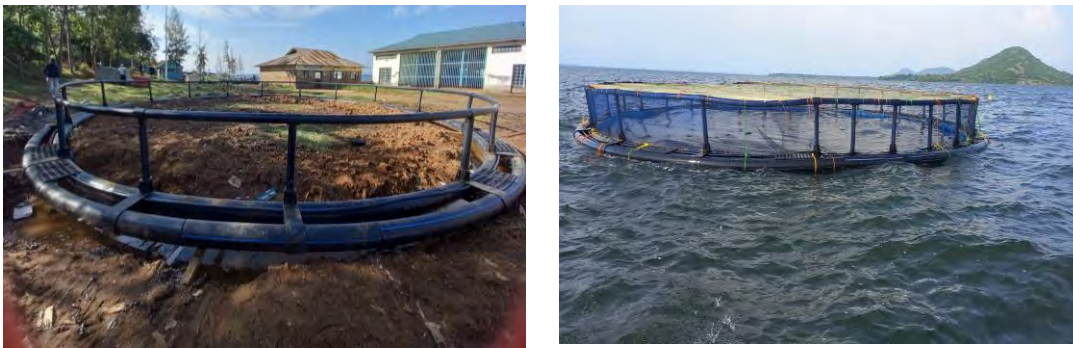
15m-HDPE fish cages constructed in Anyanga and Mulkoba beach in Siaya and Busia Counties, respectively
